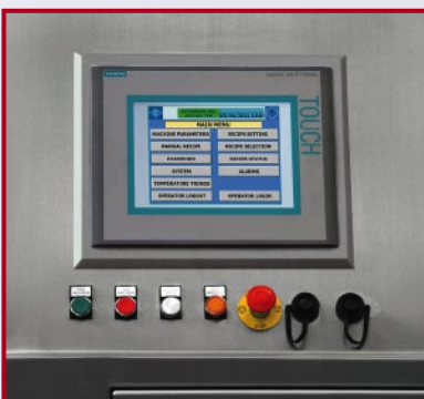
Pannello operatore touch screen Touch screen control panel
